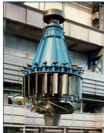
Fig. 3. The turbine upper cover with the guide vane assembly and the rotor is being lowered, Datong project China
